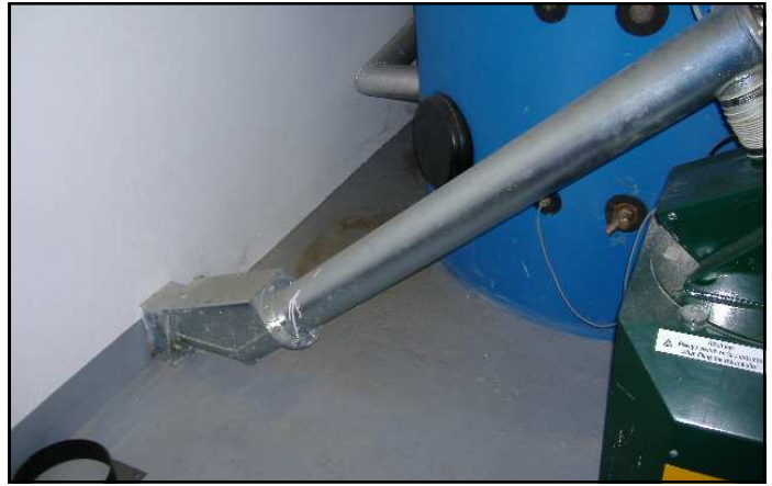
Above; Auger transferring the pellets through the wall into the boiler.
